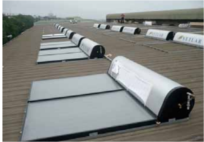
Solar heater system (Photo courtesy: Mai Huy Tan)
