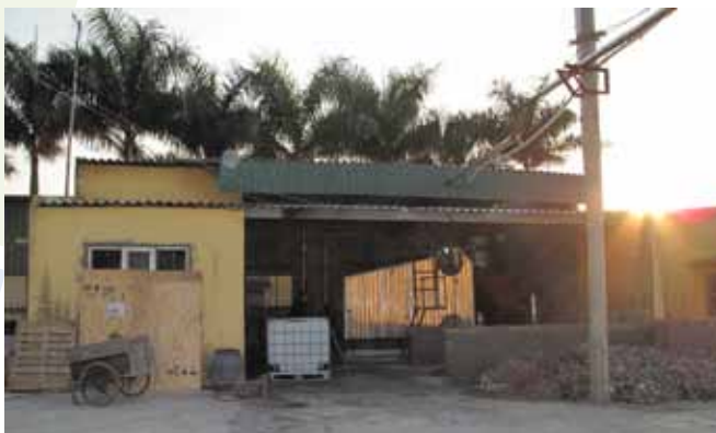
Old coal boiler to be replaced
