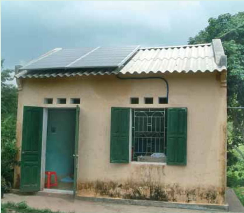
Solar panels provide electricity in Ai Quoc commune in northern Vietnam.
